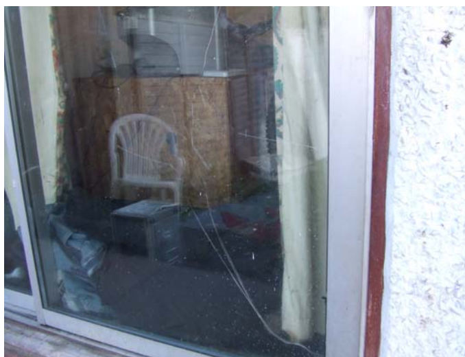
Cracked glazing to patio doors
